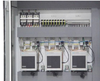
Motor control panels with 3-phase disconnect
